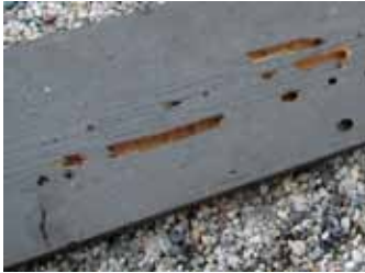
Figure 2.39 Carpenter bee galleries in structural wood.
